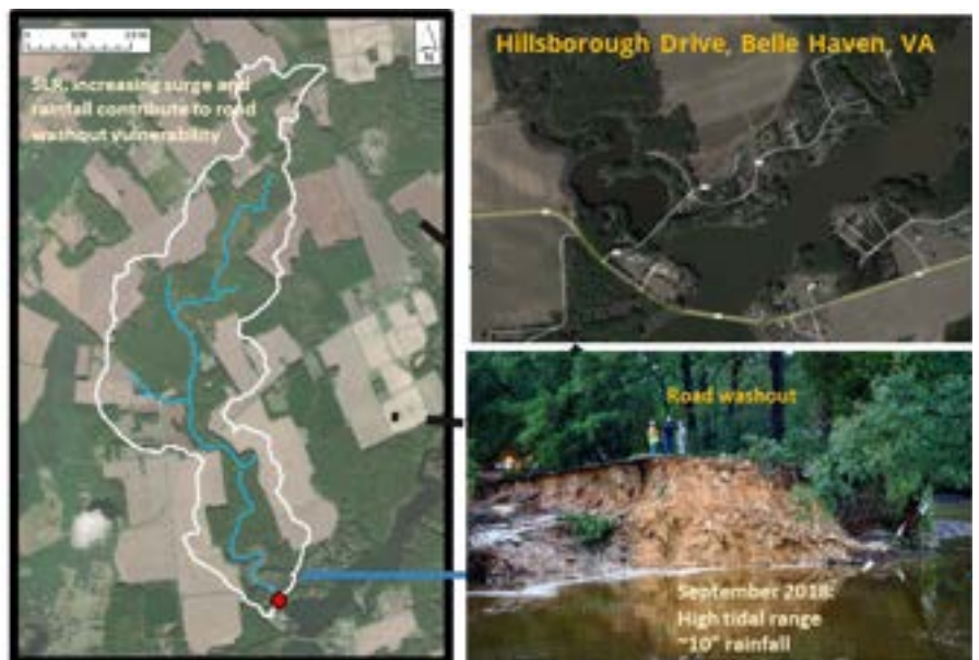
Road Washouts and Flooding
